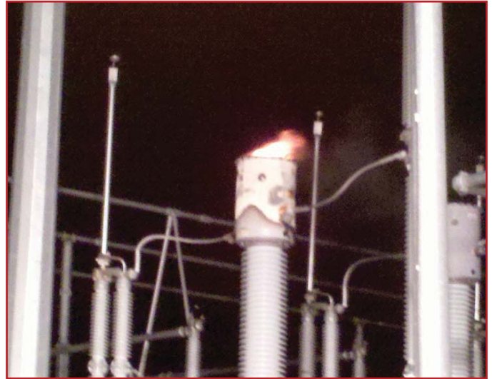
Transformer Fire After Flash
